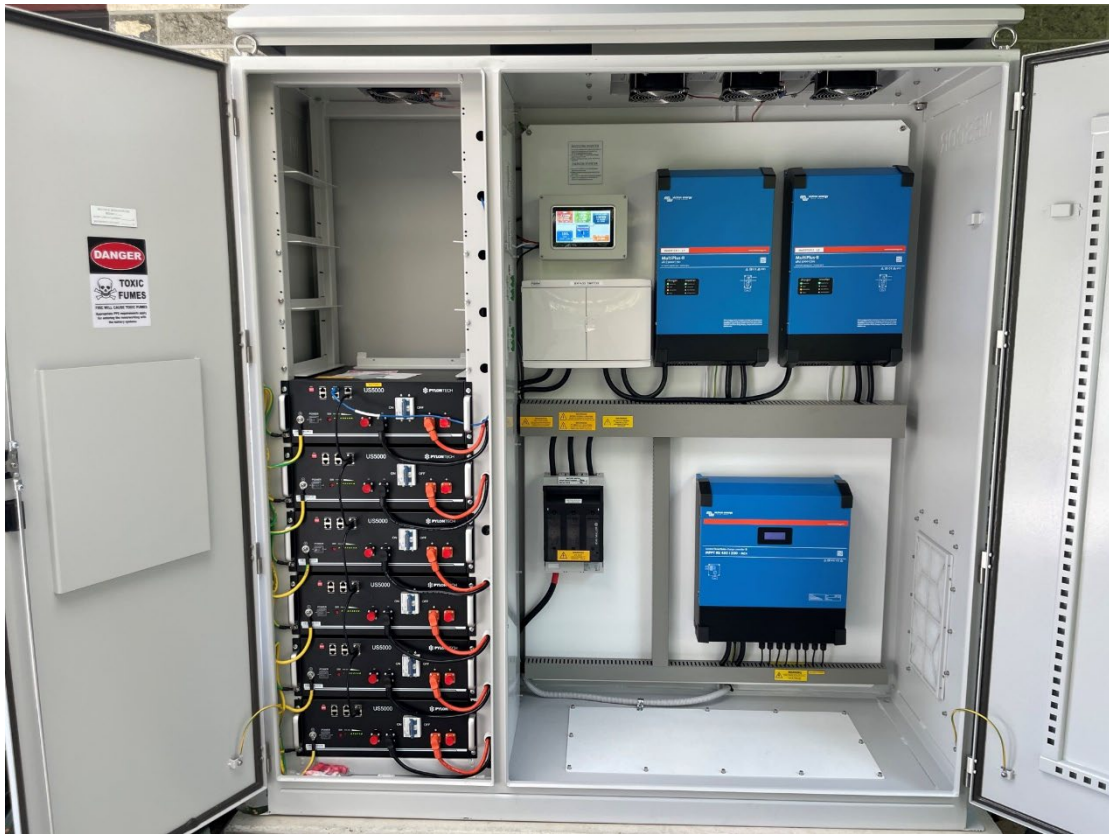
Figure 22 – Typical PCE arrangement
