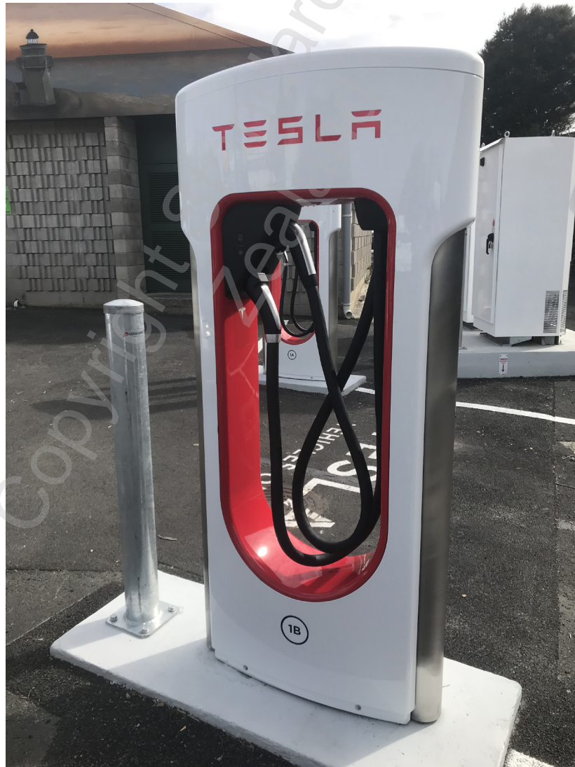
Figure 5 – An example of a bespoke EV charging station
