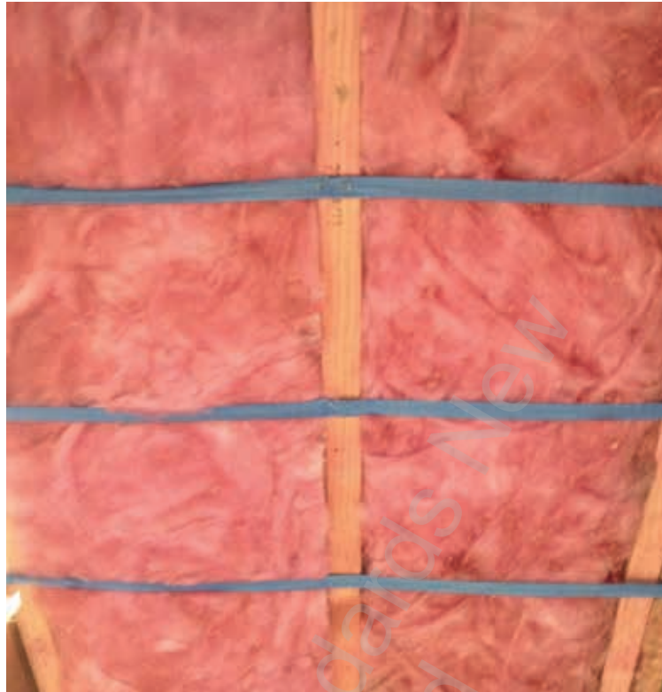
Figure 28 – Blanket in a ceiling secured with strapping
