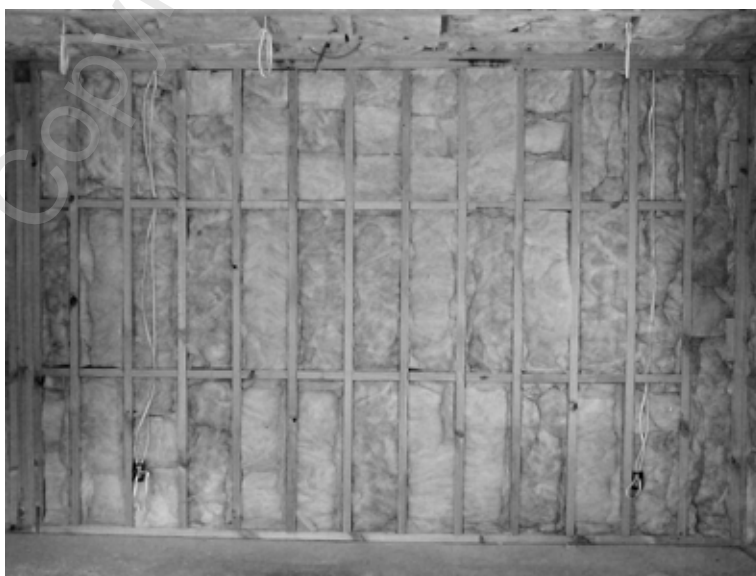
Figure 1 – Insulation installed with gaps, tucks and folds
